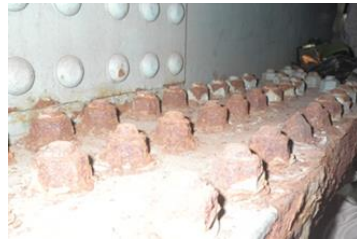
Fig 1. Corrosion of joint
