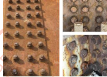
Fig. 1 Corroded high strength bolt connection
