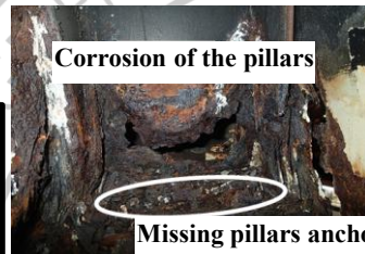
Fig. 2 Damage of steel parapet
