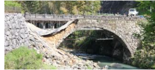
Fig. 1 Examples of damage (Kumamoto earthquake)
