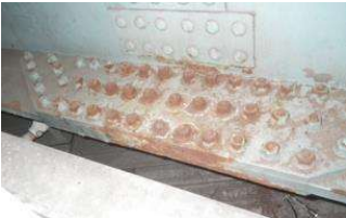
Fig.1 Corrosion of joint
