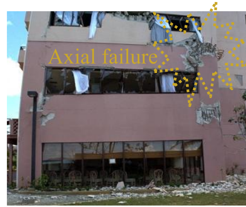
EQ damage from Guam Island Earthquake in 1993
